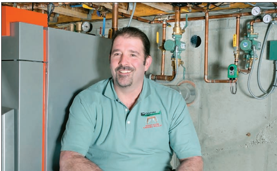
Steve Gronski prefers Taco Viessmann boilers and Taco pumps and related equipment on his radiant heating jobs.
