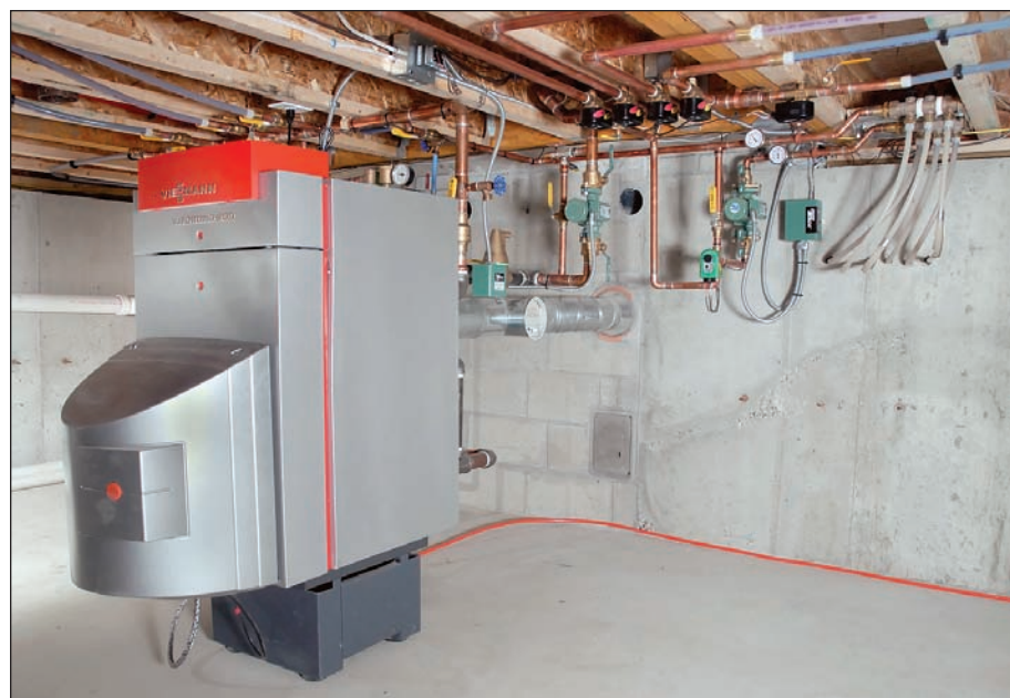
The complete heating system includes a Viessmann Vitorond boiler, a variety of Taco circulators, valves and controls, and a SuperStor Ultra indirect water heater (not shown).
