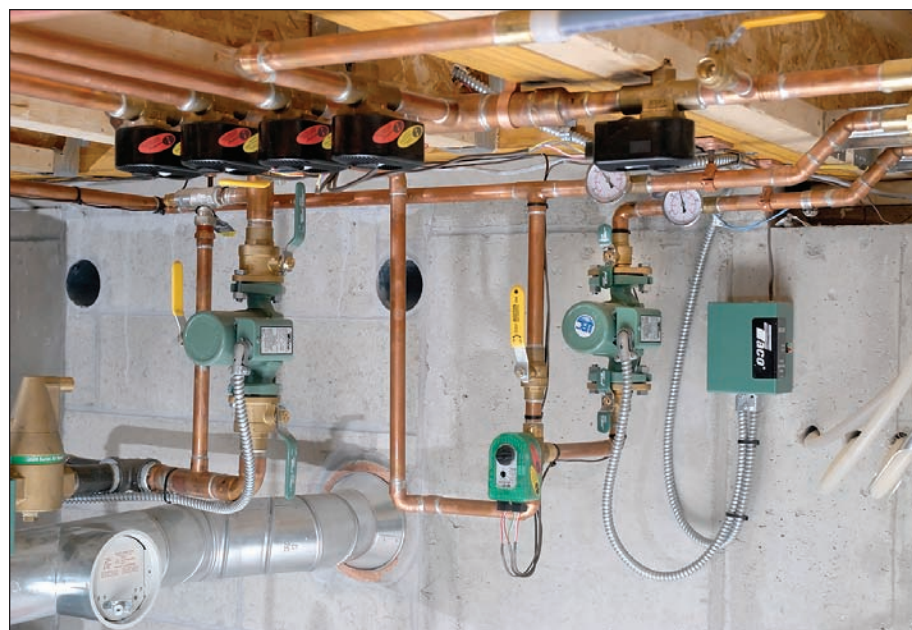
Close-up of the array of Taco equipment includes "00" circulators, iSeries Valves, EBV zone valves, an SR501 relay, a residential 4900 Series air separator and a Freedom flange.
